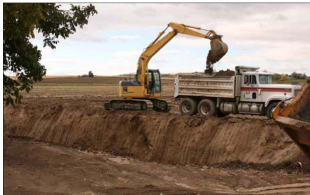
Figure 1. A constructed sedimentation pond will collect irrigation tailwater for reuse on the farm.
