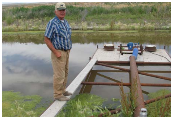
Figure 4. Jerry Wilcox of Vale, Oregon demonstrates a pump on a float in a sedimentation pond on his farm. The float is hinged at the bank of the pond so that the float always keeps the pump at the proper height above the water level.
