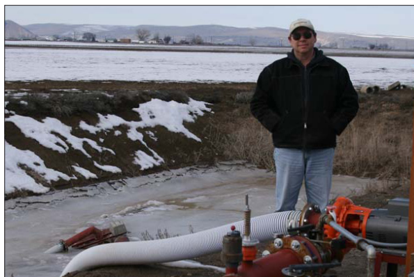
Figure 2. Intake pipe, motor, and pump for pumping water from the pond back into the irrigation system.
